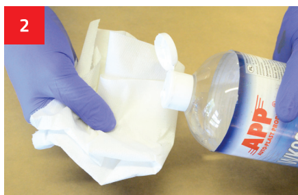
2 Before starting the repair, the surface should be cleaned and degreased using WK900.
